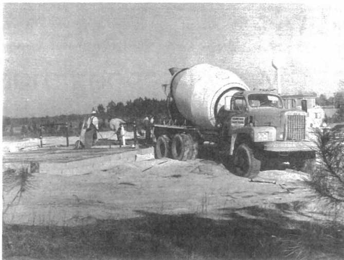
Pouring of concrete for a new residence cottage was a sign of progress at the Boys Ranch near the end of 1979.
