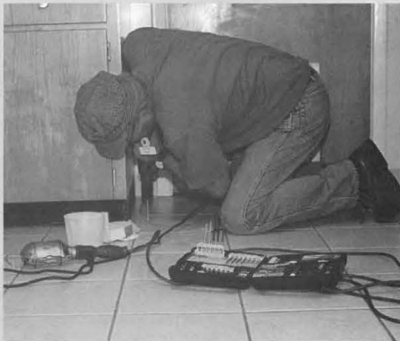
Jim Rhodes of Indiana drills a hole to install a door stopper that will protect the kitchen cabinets from damage.
