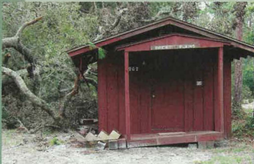
At the Youth Camp in Barberville, Hurricane Charley brought a tree down that shifted this cabin right off its foundation. Significant tree damage occurred throughout the camp.
