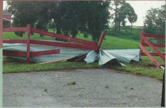
At the Youth Villa in Bartow, Hurricane Charley tore part of the roof off the barn and blew it right into the fence. Fortunately, the debris did block the fence line and the horses remained in the paddock.
