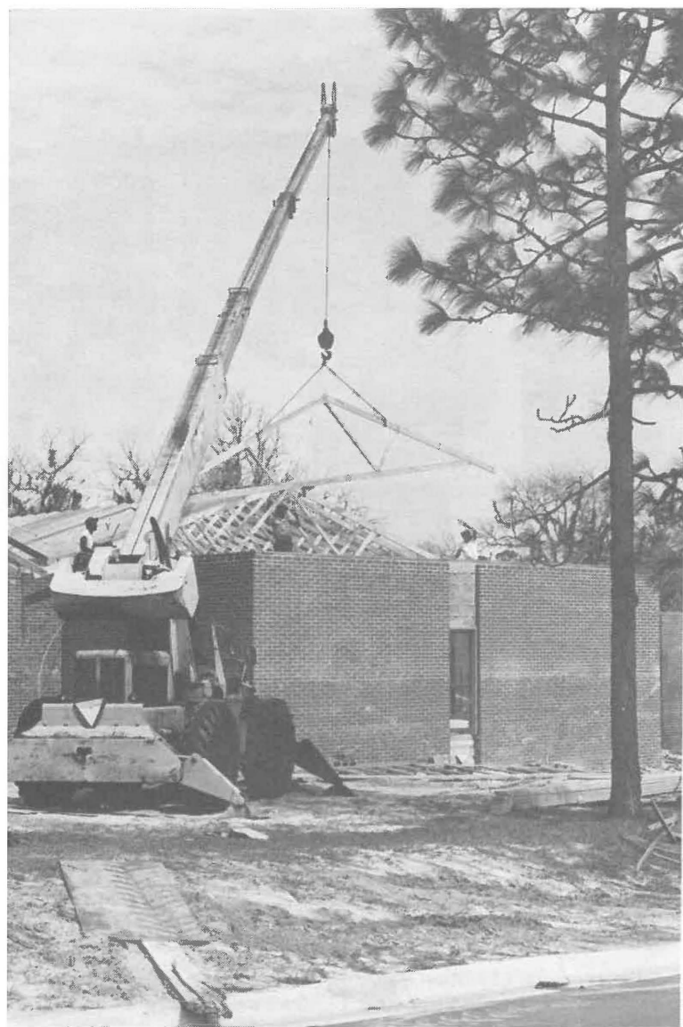
In a matter of months, the new education center will be ready for occupancy.
