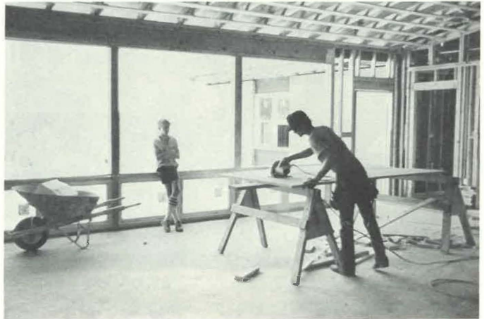
The Boys Ranch will be 20 years old on October 2, but it's still growing. Workmen are putting the finishing touches on Jellison Cottage, newest residence cottage on the campus.
