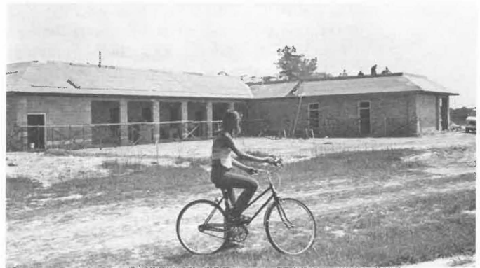
Workmen are making speedy progress on the Girls Villa activities building. Its facilities will include a recreation area, a learning center, a chapel, offices and a swimming pool.
